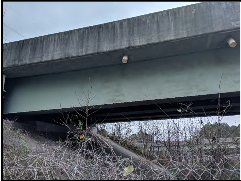
5 Expansion joint located on concrete retaining wall and the joint at the slope and foot tested negative for asbestos via PLM and TEM analysis.
