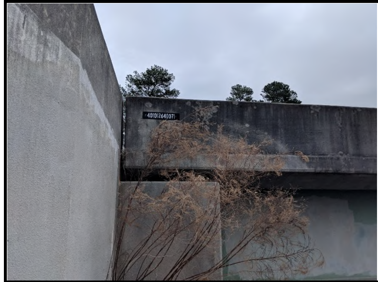
4 Textured coating located on retaining wall tested negative for asbestos via PLM analysis.
