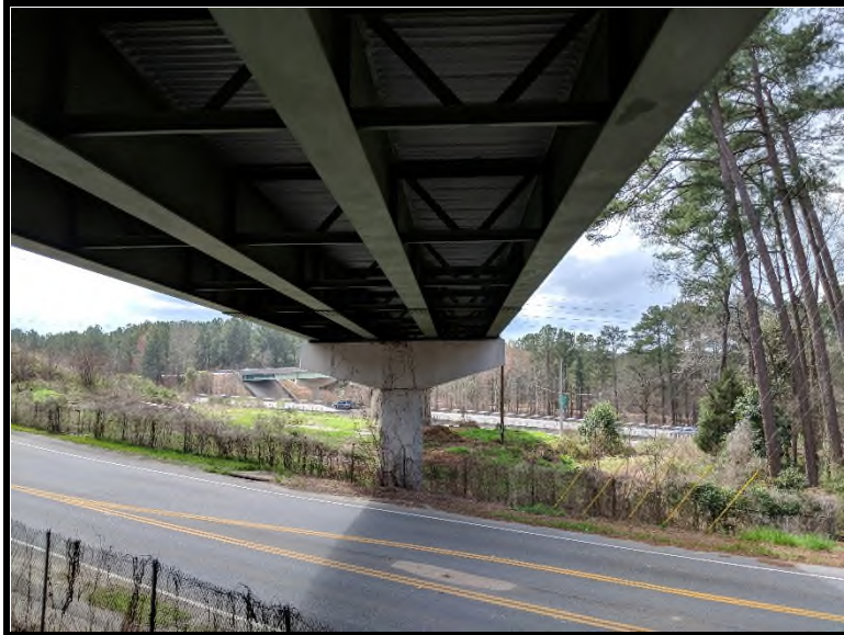
3 View of the underside of the bridge. Shows steel beams, metal decking and concrete piers.
